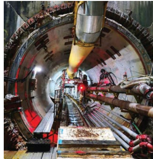
Murname Pipeline Project Package 5 Water Transmission Pipeline (AYE / Henderson Rd to River Valley Rd)
